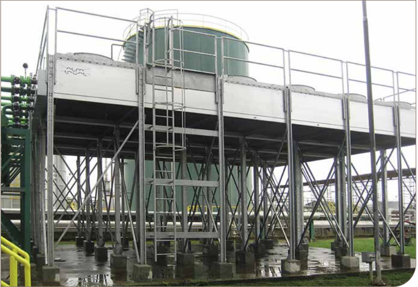
FBL fan cooler typical installation including steel structure, ladder and handrails
